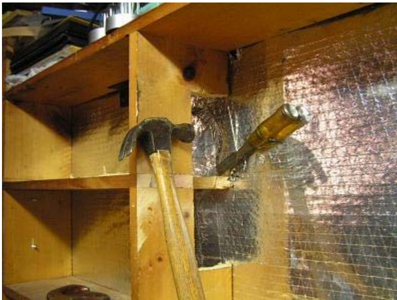
Figure 17 Using a hammer and chisel to notch out the cable access hole
